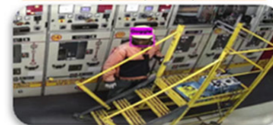
PPE noncompliance detected by system (Safety Goggles)
