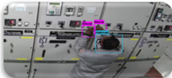
PPE noncompliance detected by system (Helmet)
